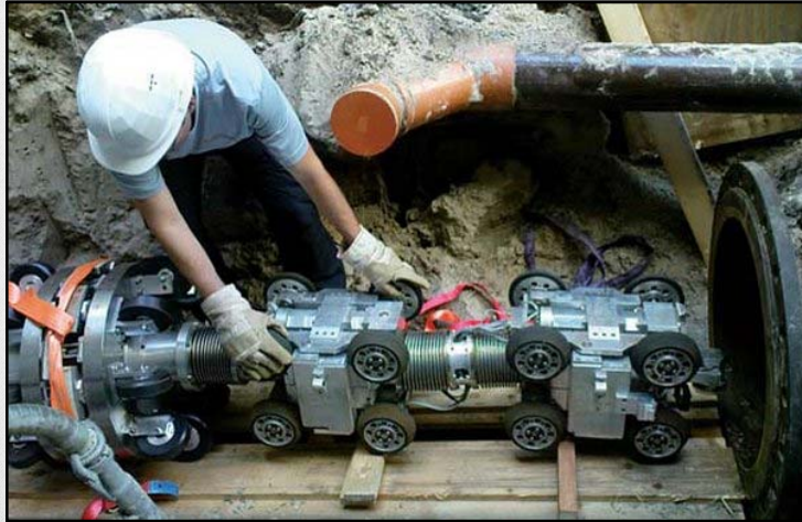
Robotic Coolant Pipe Inspection
