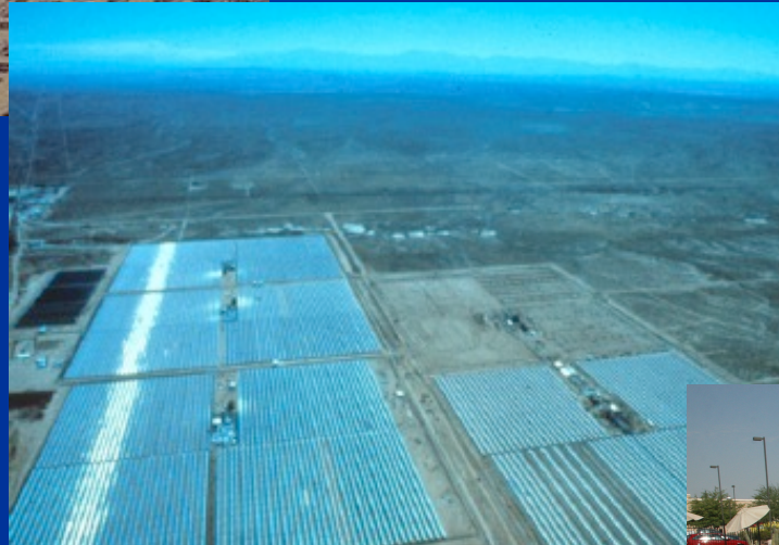
350 MW Parabolic Trough Power Plant, California
