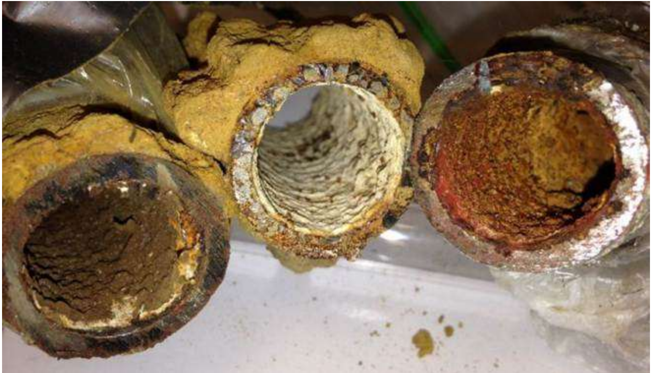
Corroded pipes from Flint's water distribution system. Credit: Min Tang and Kelsey Pieper
