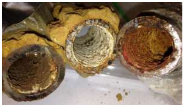
Corroded pipes from Flint's water distribution system. Credit: Min Tang and Kelsey Pieper
