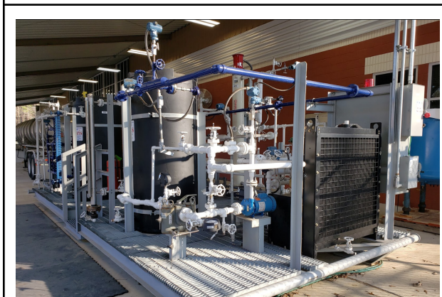
HOT Skid Unit
