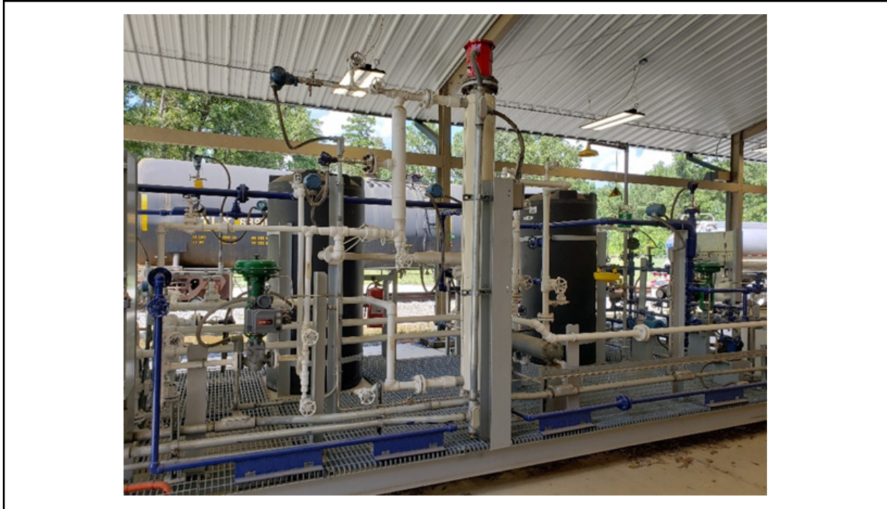
HOT Skid training unit at South Ark CC.
