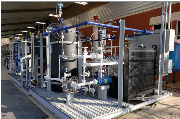
HOT Skid Unit
