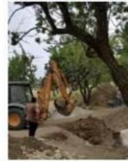
Figure 6. Workers removing a wall around the site because it was found to be a Roman wall. The wall was found to be a Roman wall. (Photo: Jonathan Broda)
