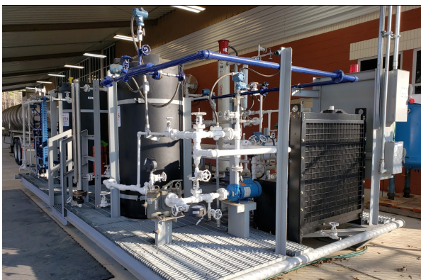
HOT Skid Unit
