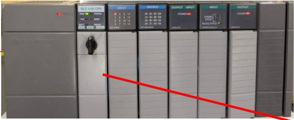
SLC-500 chassis, power supply, processor & I/O modules
