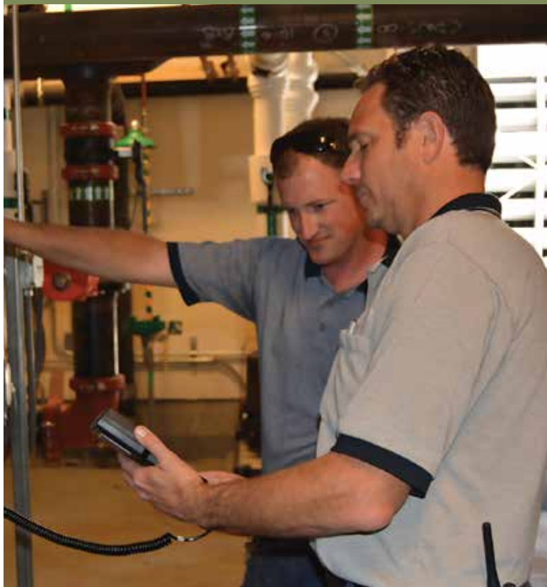
Technicians inspect a commercial chiller to repair or replace components before failure occurs.
