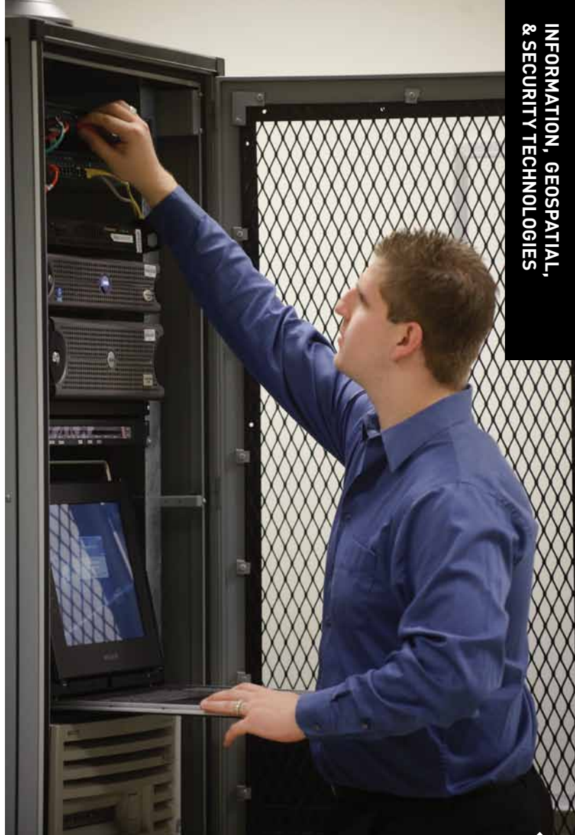
A CSSIA GRADUATE MAINTAINS AND SECURES A DATA CENTER.
