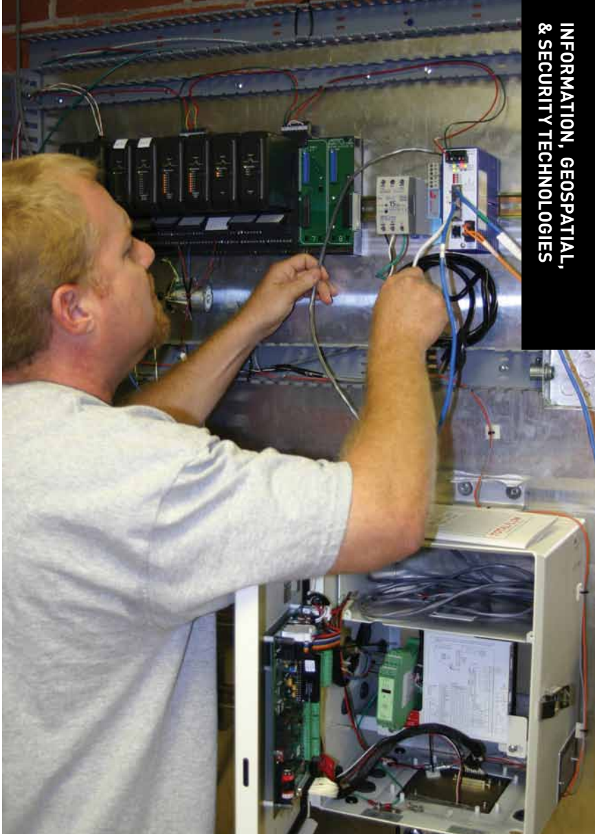
A TECHNICIAN TROUBLESHOOTS A PROGRAMMABLE LOGIC CONTROL SYSTEM AND ASSESSES ITS CYBERSECURITY ATTACK VULNERABILITIES.
